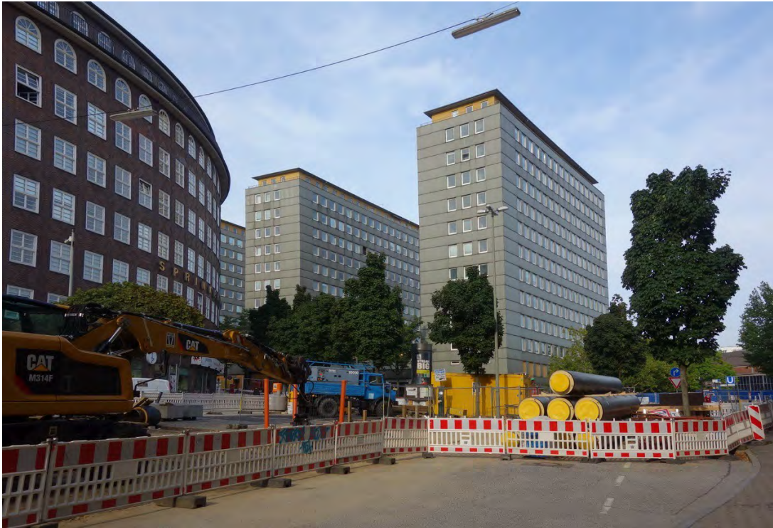
Fig. 10. The surroundings of the Johanniswall and Burchardstraße (partly territory of the World Heritage property and the buffer zone). Present state of the City-Hof prepared for demolition. Photo: N. Dushkina, 30.08.2018
